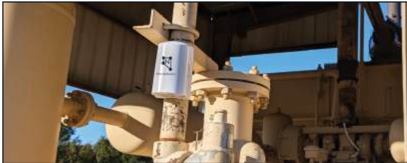
MethaneTrack™ wireless sensor mounted in close proximity to compressor
