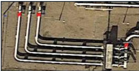
Leak locations confirmed
