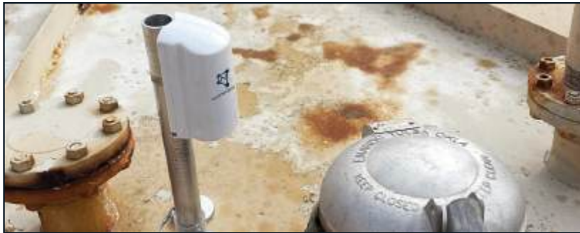
MethaneTrack™ wireless sensor mounted on tank near thief hatch
